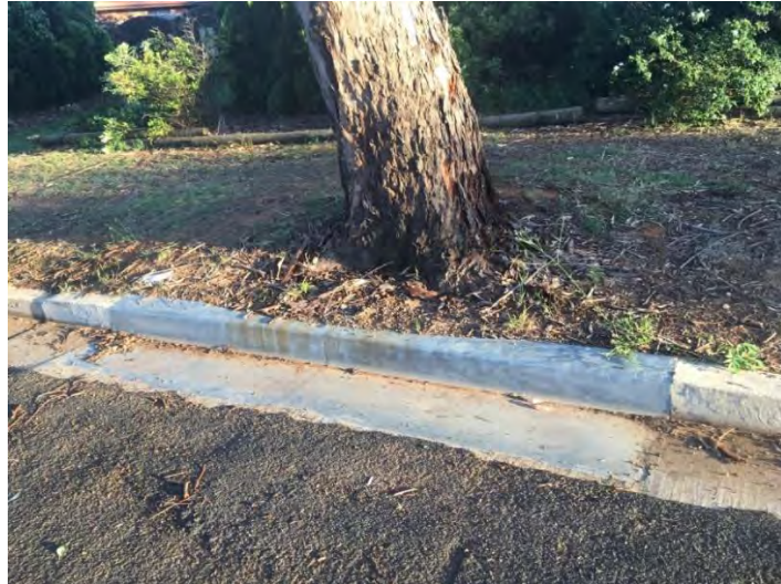
Photograph 10. Retention of Eucalyptus robusta at Bellbird Way through the installation of a formed steel gutter over the structural root zone.
