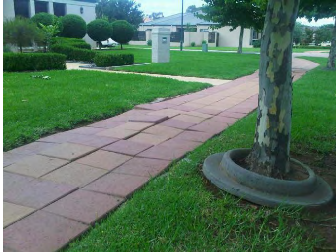
Photograph 3. St Andrews Drive showing damage to segmented pavement by tree roots.
