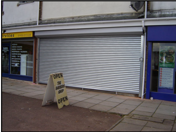
Photograph 10: Security grille type which is considered to detract from the business and the street
