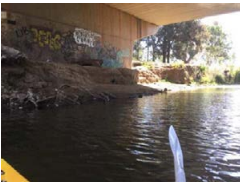
Figure A6.6 erosion scarp.
