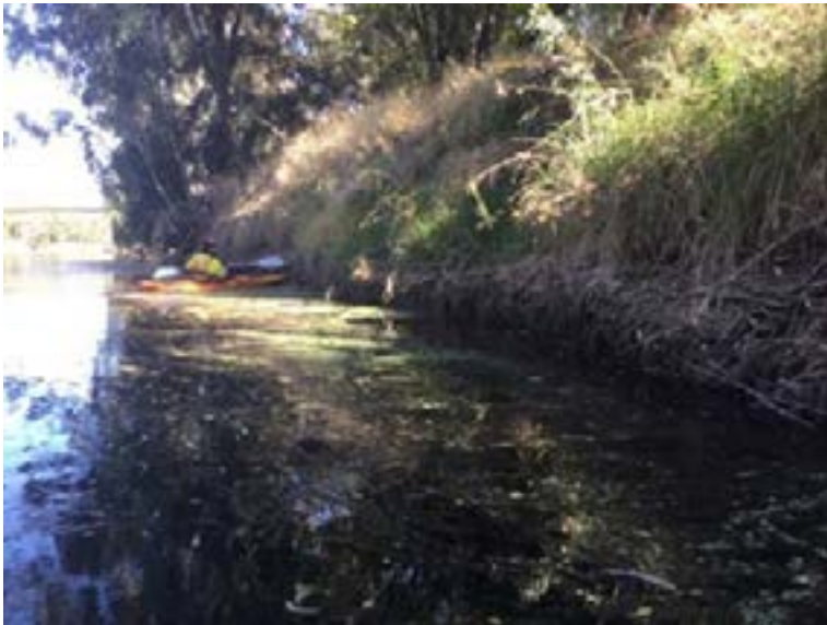
Figure A6.5 bank erosion
