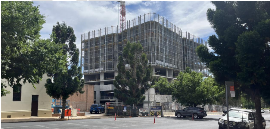
Figure 17: 1 Church Street, Dubbo, November 2024
